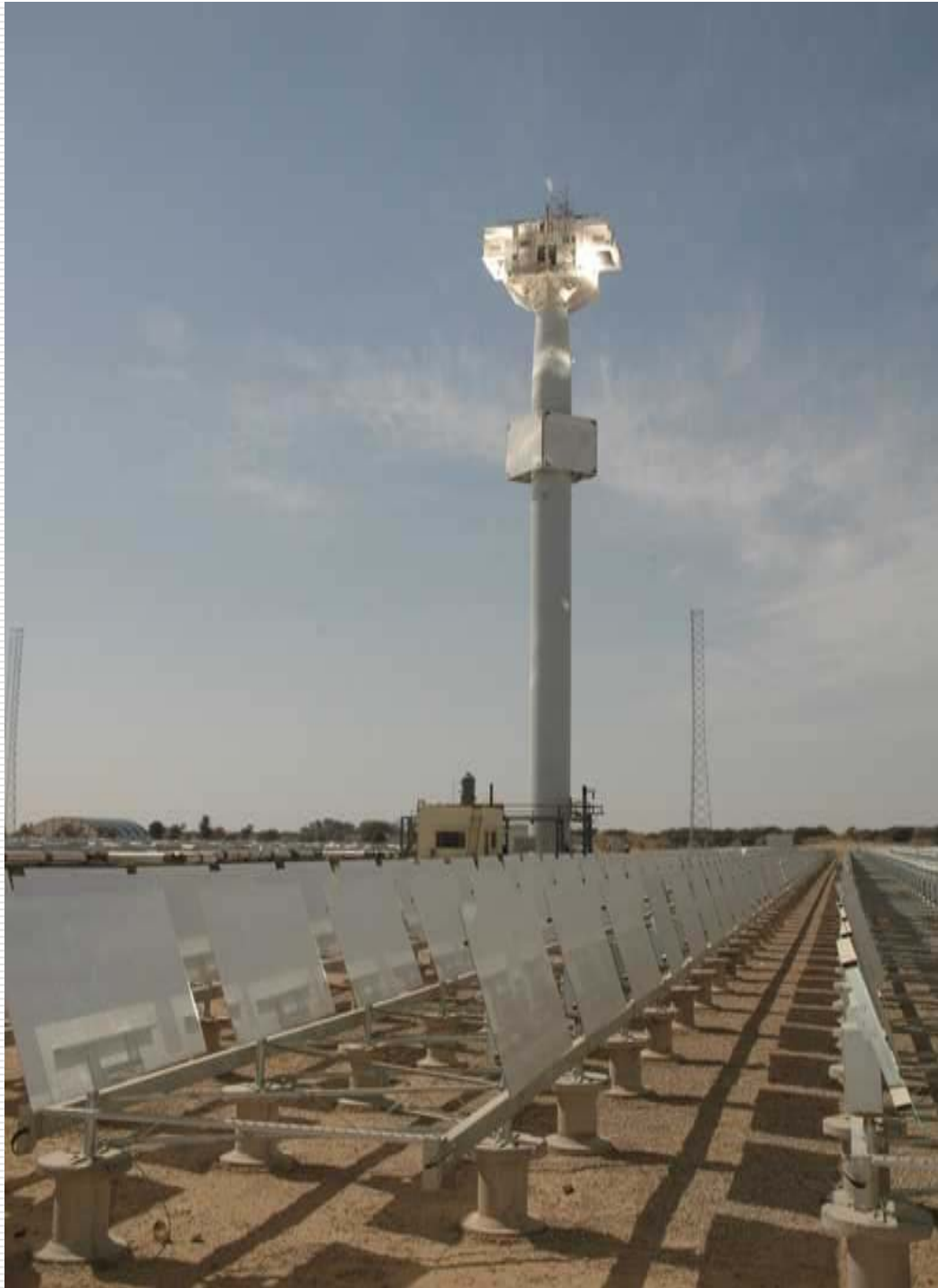
2.5 MW Solar Thermal Tower Grid Power Plant at Bikaner, Rajasthan
