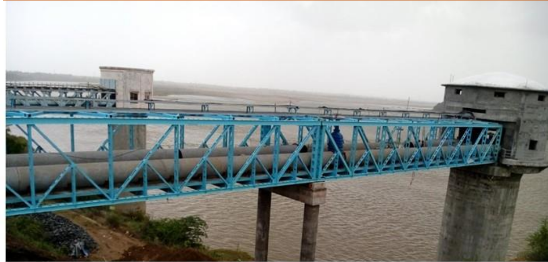
Intake Wells : 227 MLD on Narmada River
