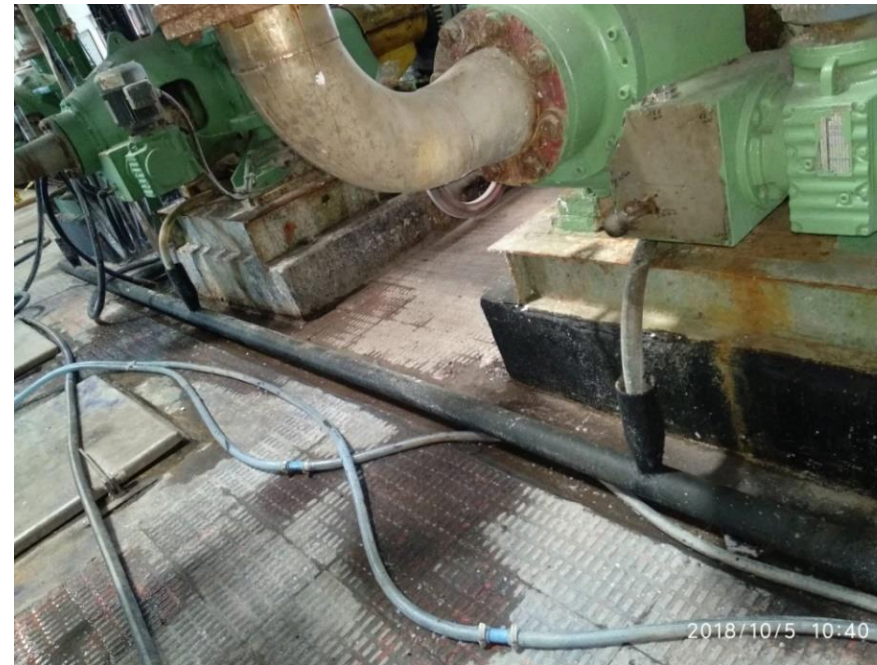
After - Pump Seal Cooling Water Collection system
