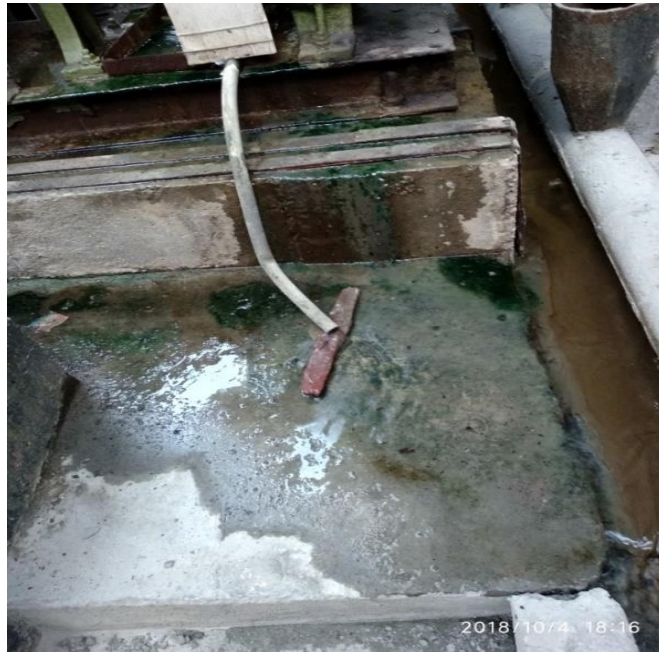
Before- Seal cooling water going to drain
