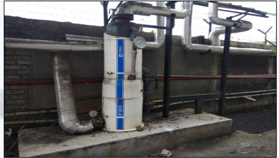
CONDENSATE RECOVERY SYSTEM at ULTRA DENIM
