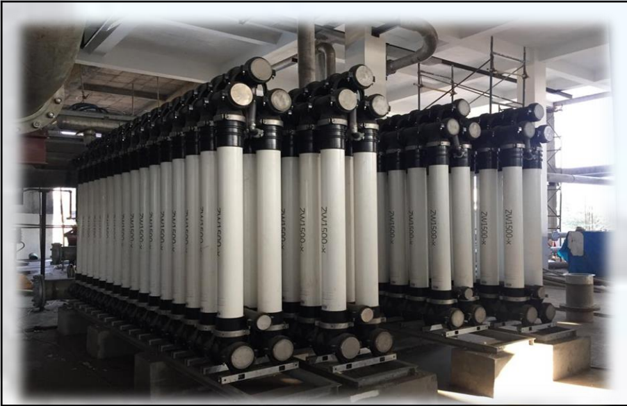
RECYCLING PLANT - UF SKIDS – 6 MLD
