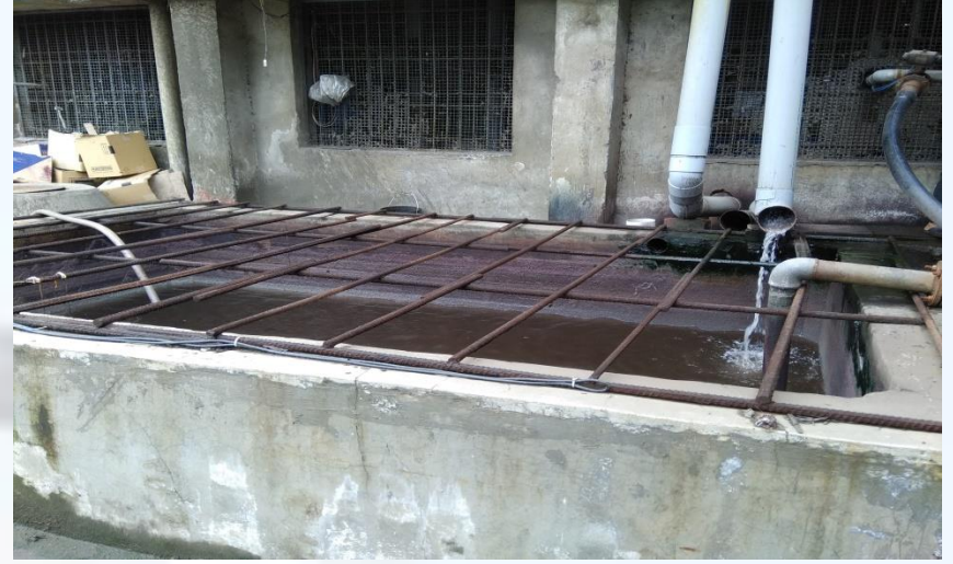
ETP COLLECTION TANK and Reuse at VIRAJ
