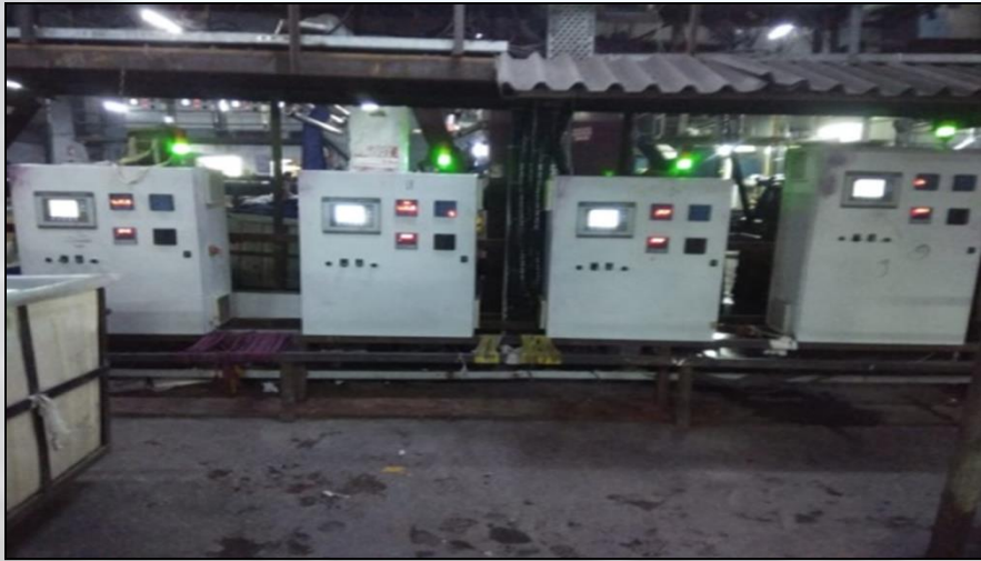
U JET M/C PLC PANELS at GINZA INDUSTRIES
