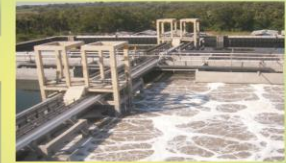
Common Effluent Treatment Plant
