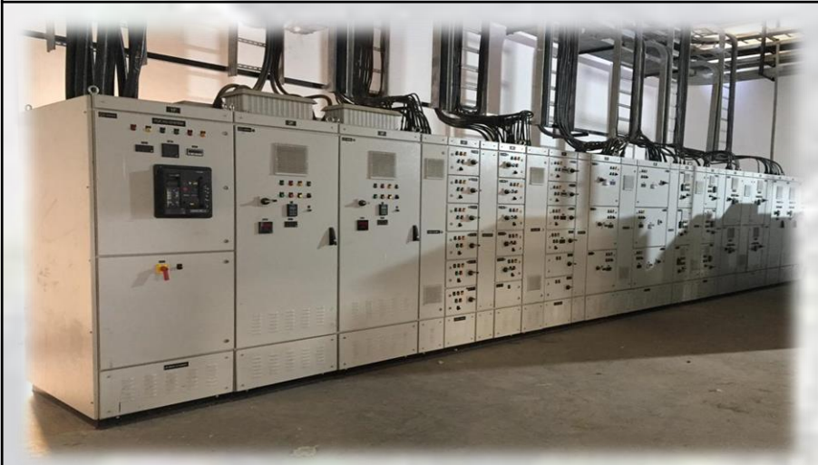
ELKECTRICAL PANELS for UF/RO
