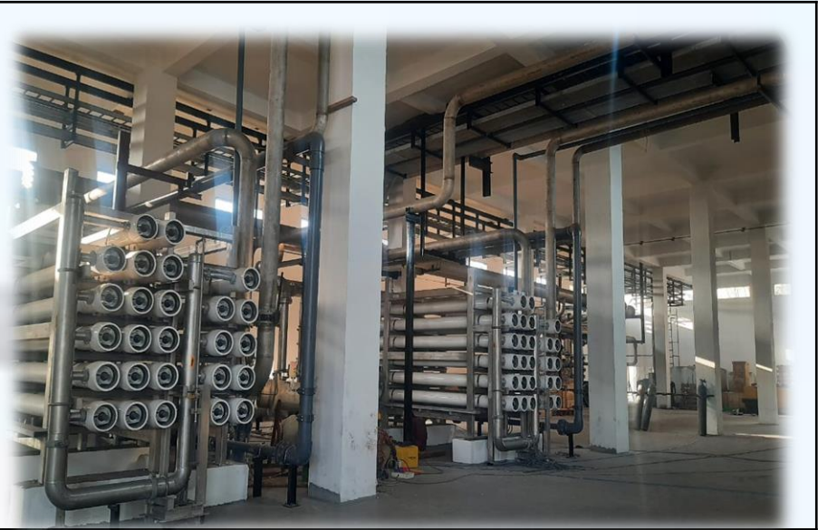
RECYCLING PLANT - RO SKIDS – 6 MLD SKID
