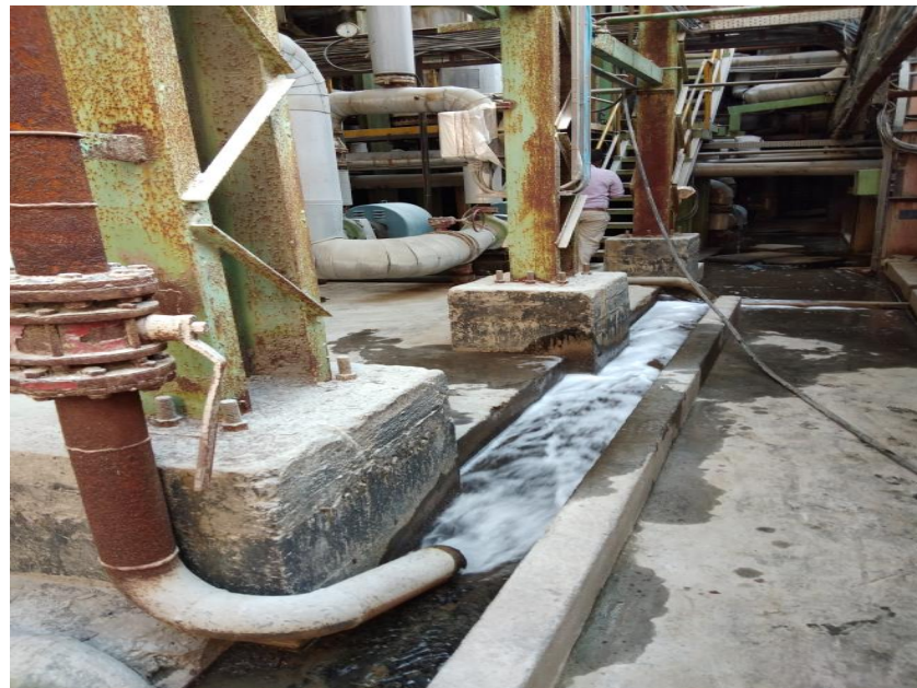
Secondary Condensate drained from Evaporator Section to ETP
