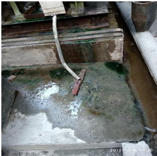
Before- Seal cooling water going to drain
