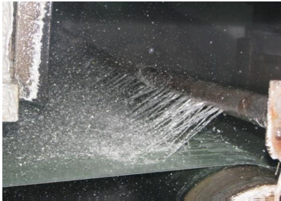
Fig 3: Inefficient Hole Showers consuming more water
