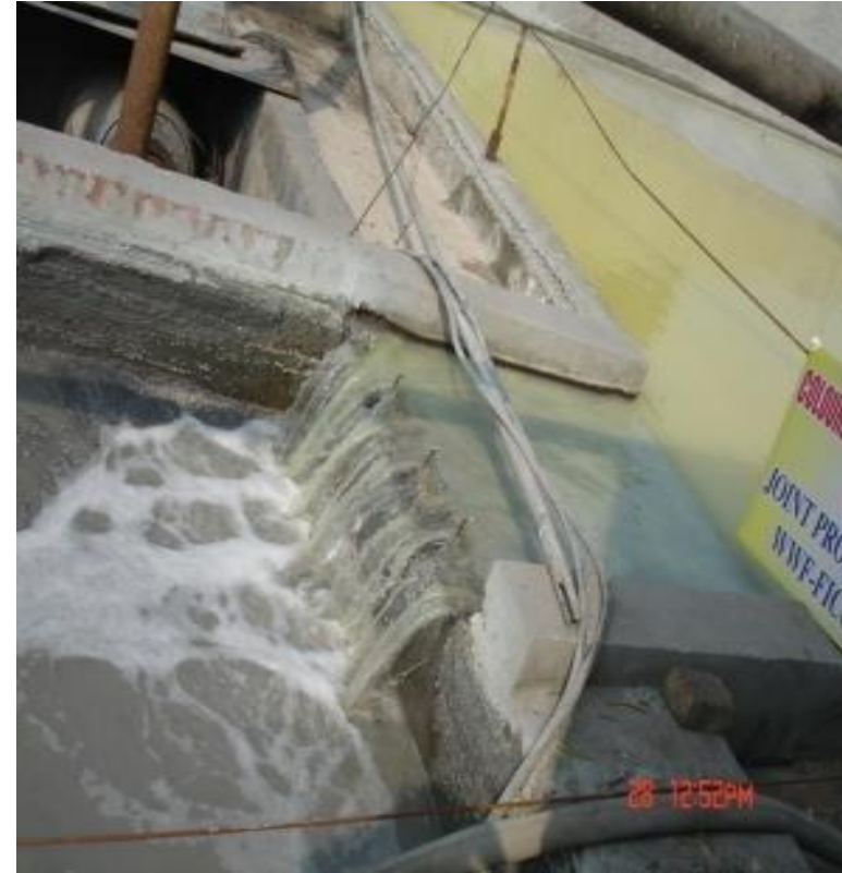
Treated Effluent Discharged to common pit
