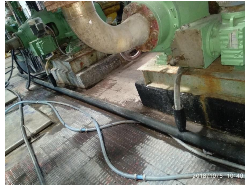
After - Pump Seal Cooling Water Collection system
